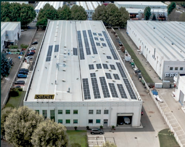
Clean energy production from solar panels
